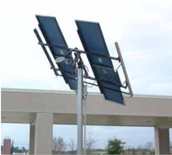
New 600 Watt Solar Array
